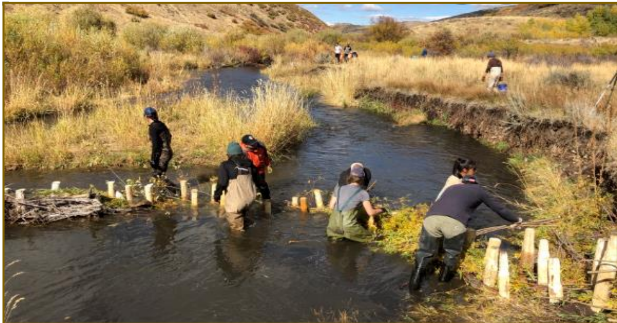
BDAs being installed in East Canyon Creek, Wasatch Mountains area, Utah. Photo by Mark Edgley
